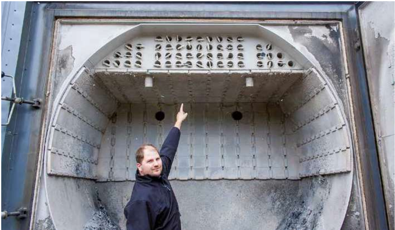
The smoke pipes at the top of the boiler must be cleaned every 14 days. Otherwise there isn't much maintenance.
